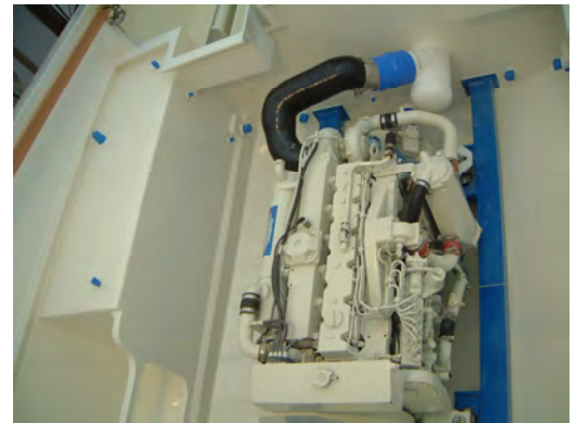
Engine room constructed using plastic honeycomb +18 oz WR panel system for sound and vibration absorption.
